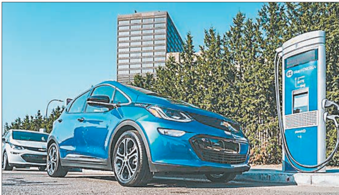
This EV charging station was recently placed in the downtown neighborhood of Beacon Park in Detroit.
