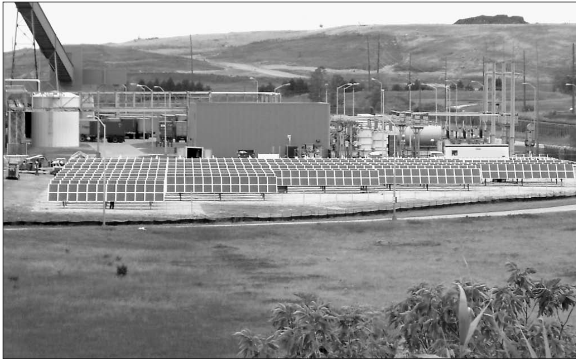
Solar Panels at Orion Assembly helped GM save on energy costs, meet EPA's ENERGY STAR Challenge.
